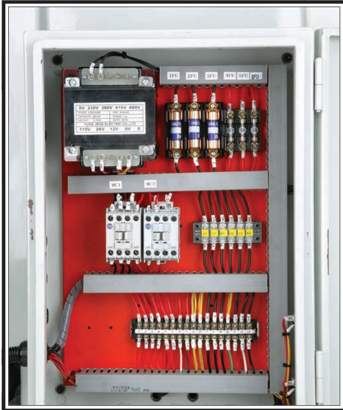
Figure 72. SB1025 Electrical box.
