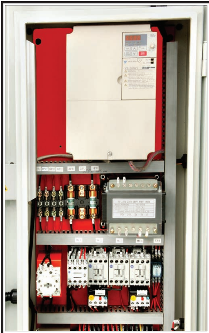
Figure 69. Electrical cabinet wiring.
